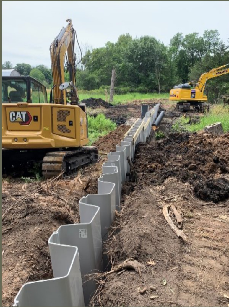
Cut off water seepage Inadequate soil for berm
